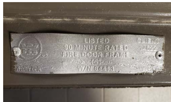
hollow metal frame
