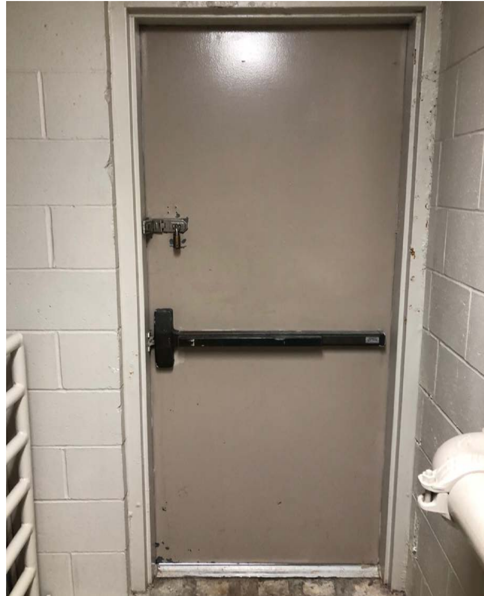
exterior mechanical door
