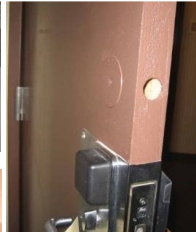
deadbolt never installed on opening
