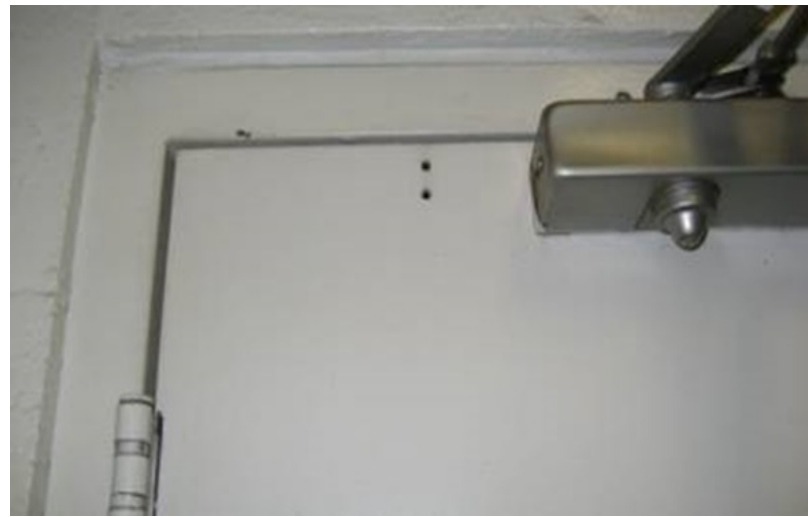
relocated closer exposing original mounting holes
